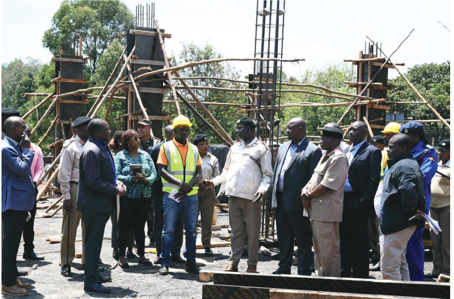
The Central Regional Implementation Committee (RICMC) at the site where a modern market is being built in Othaya constituency.
